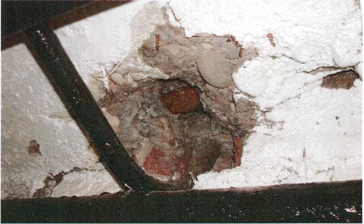
The ceiling is crumbling due to water damage.
