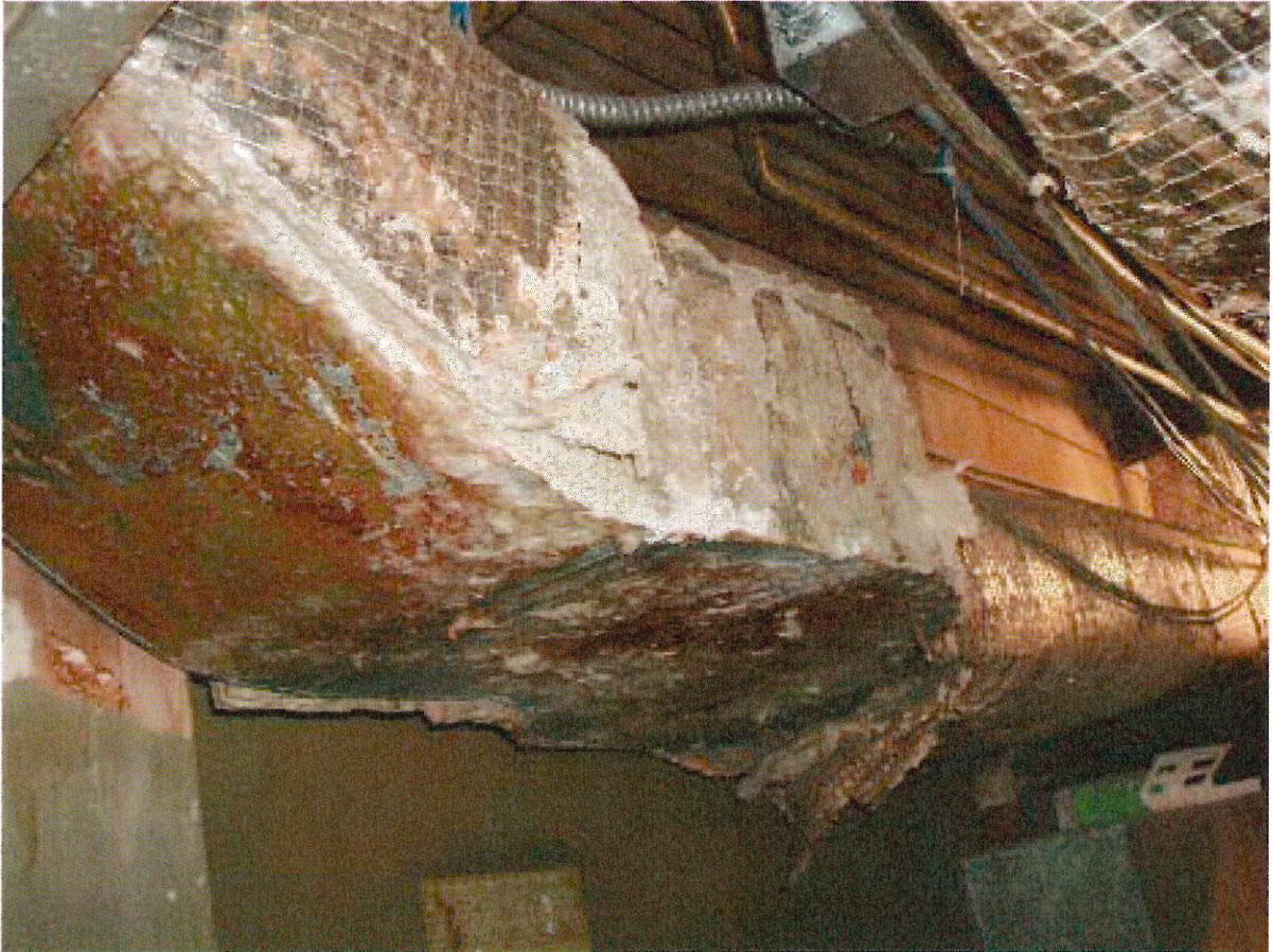
Rusting, decaying air ducts.
