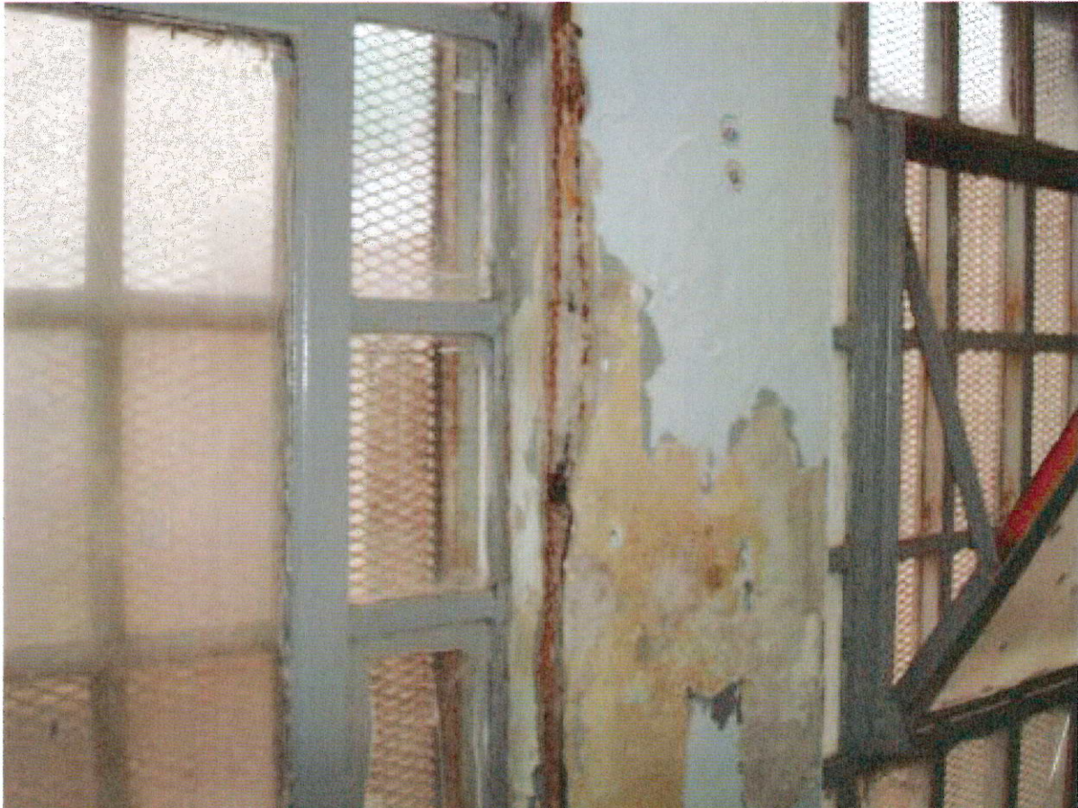
Crumbling wall adjacent to windows of a cellblock.
