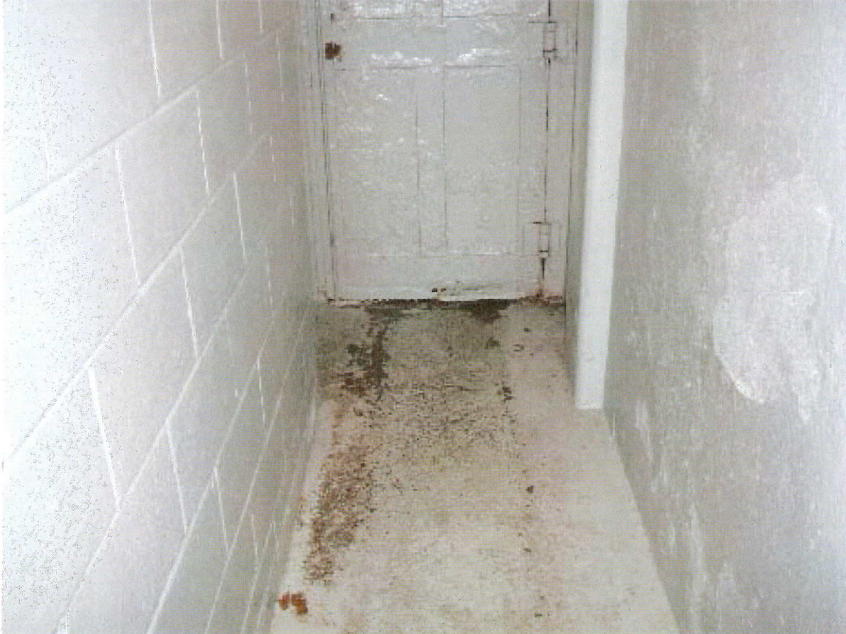
Flooding and water damage in a hallway.
