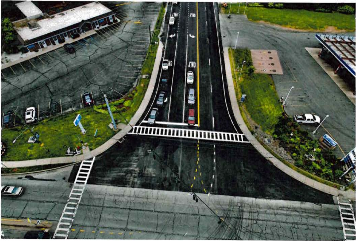
County Road 103 / State Route 42 Intersection vicinity Walmart (Town of Thompson) Milled, paved and re-stripped with extensive epoxy pavement markings (June 2024)
