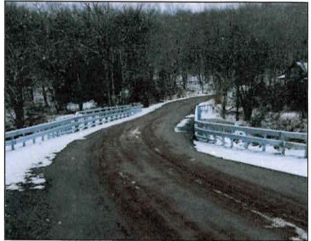
New Bridge 261 shown on Garden House Road, Liberty. Typical Example of a Bridge Designed by the Division of Public Work's Engineering Bridge Unit and Built by DPW's Bridge Operations Unit.
