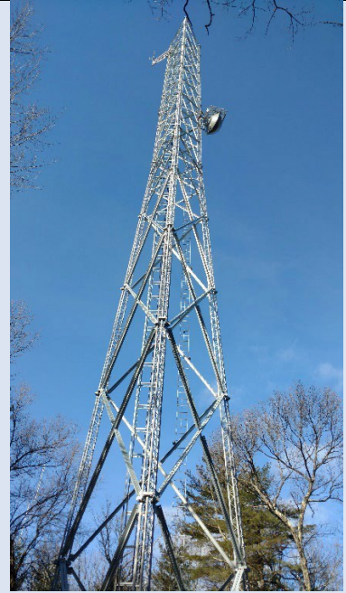
Rock Hill tower supporting not only Public Safety Communications but also Verizon Wireless equipment to enhance service. More to come in 2025
