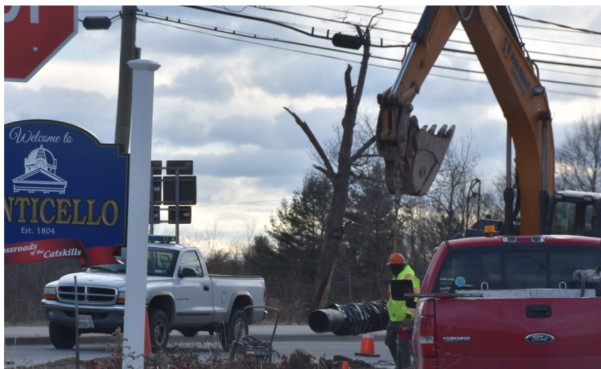
As many a traveler knows, traffic along Jefferson Street in Monticello has been delayed regularly of late due to the need to lay a water service line (seen being hoisted) from the new Sullivan County Jail to the Village of Monticello's new water tank. This line, when complete, will also be able to serve the Jefferson Street corridor.
