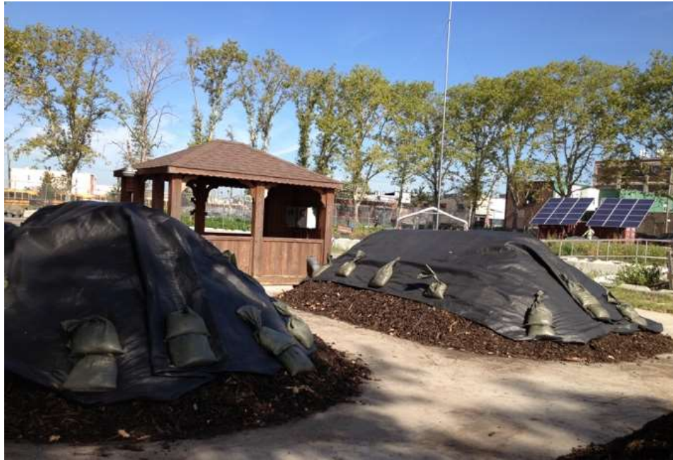
Exhibit 13. ASP System Powered by Solar Photovoltaic Array at Red Hook Community Farm, Brooklyn, NYC
