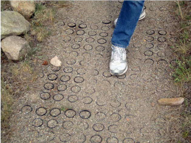
Trail surface material can be further stabilized with a variety of products (Source: National Trails Training Partnership)
