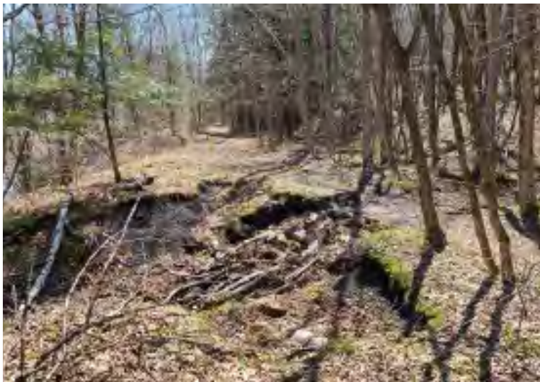
One of the existing washouts that will be addressed with a new closed drainage system.
