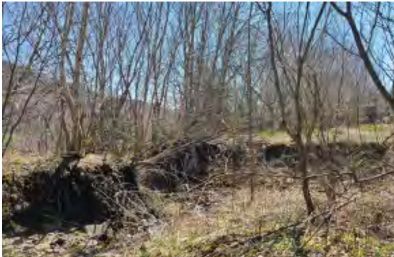
Looking east towards where the rail bed has been washed out. This area to be replaced with a box culvert.
