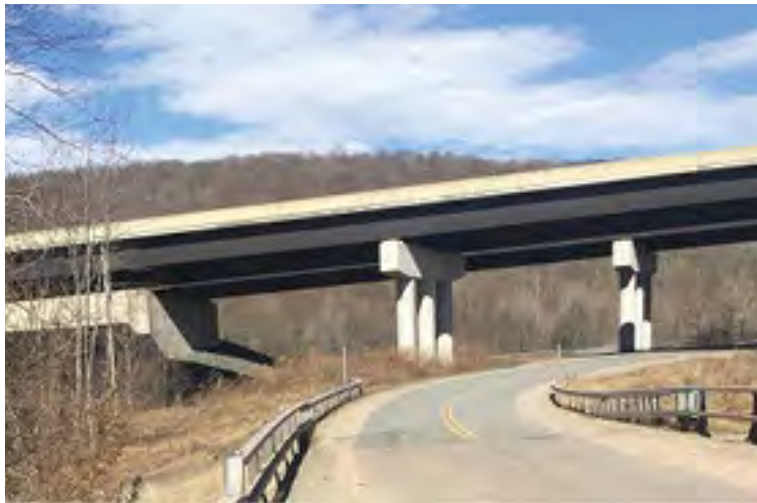
Looking northeast towards the bridge on Fox Mountain Road (BIN 2229030) over the Little Beaver Kill tributary
