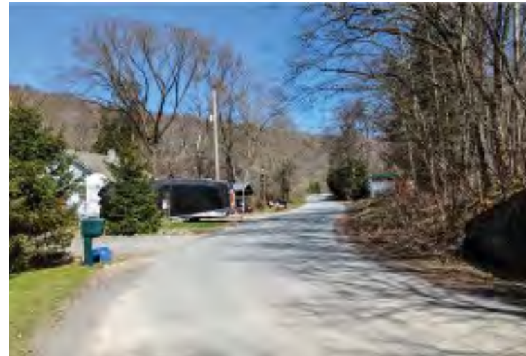
Old Liberty Road pavement distress near the bridge
