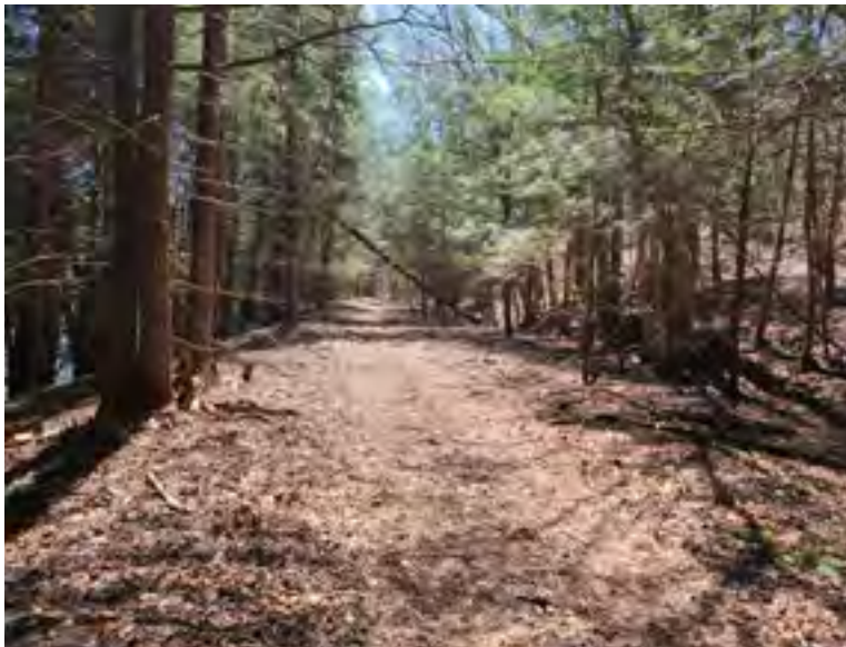
Existing rail bed beyond the washouts is consistent in grade, width, and condition
