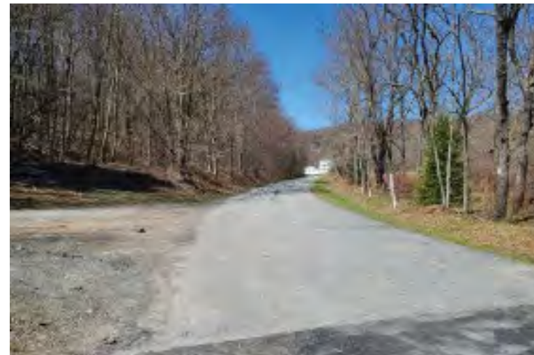
Raveling of the existing pavement is evident due to turnarounds near the Sonoma Falls gate
